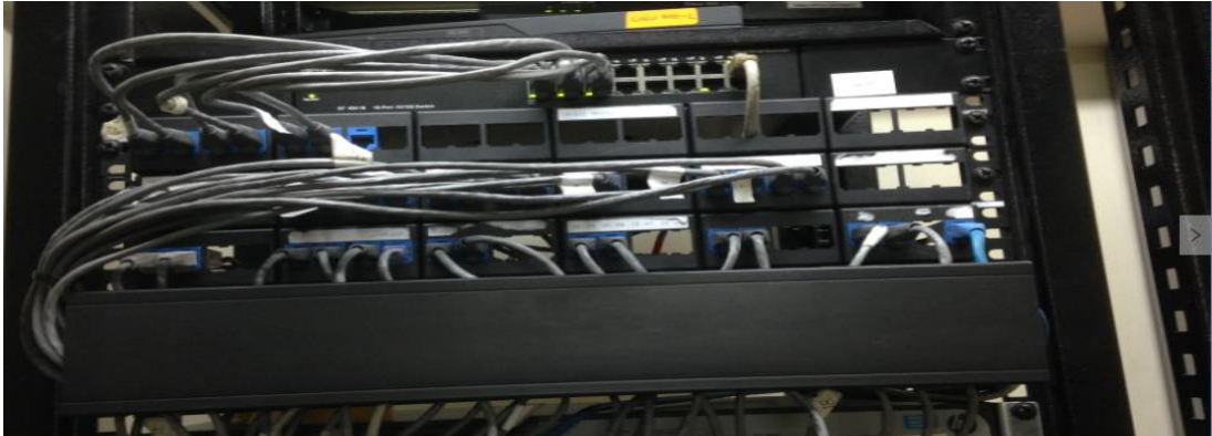
Figura 18: Patch Panel Rack
